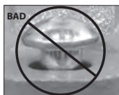
OVAL NECK OF BOLT NOT SEATED PROPERLY
