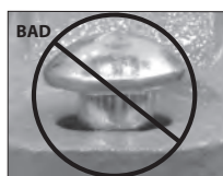
OVAL NECK OF BOLT NOT SEATED PROPERLY
