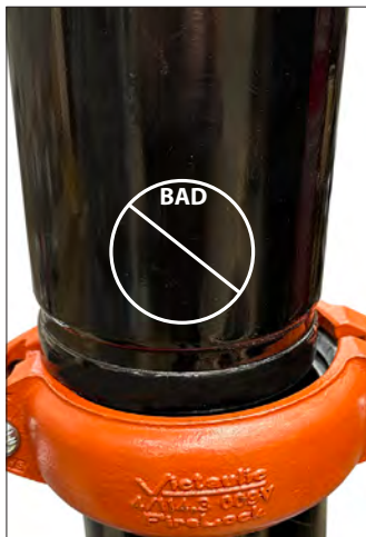
PHOTO 2 (UNACCEPTABLE) – PIPE HAS DISLODGED COUPLING
