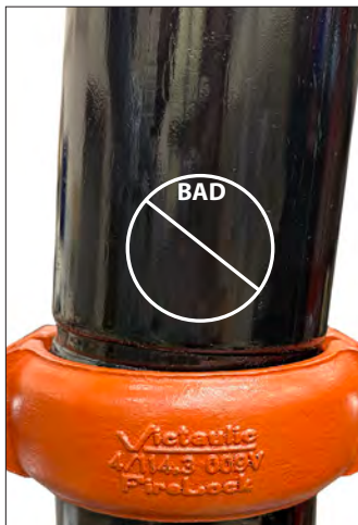
PHOTO 1 (UNACCEPTABLE) – EXCESSIVE INSERTION ANGLE
