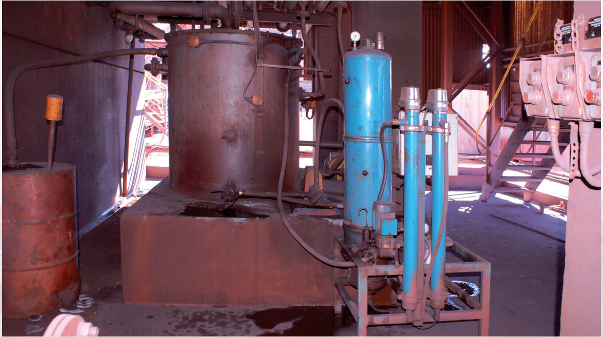
A CJC® Filter Separator installed on one of the crushers at Kumba Iron Ore's Sishen Mine in the Northern Cape, South Africa
