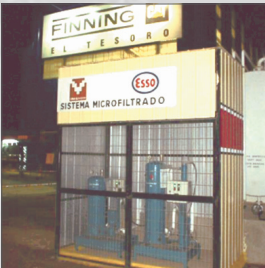
CJC® Oil Filters installed on storage tanks, Minera El Tesoro Chile
